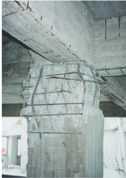
Figure 1: Column damaged during Kocaeli Earthquake Turkey, 1999 due to ineffective confinement [16]
